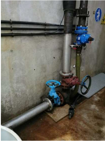
Vannes et bypass
